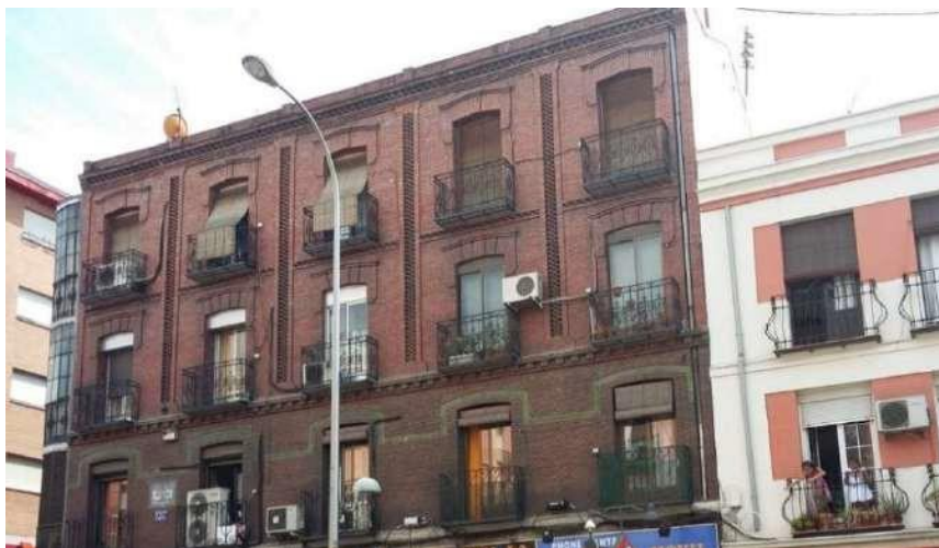
Figure 5.60. Top: Example of the proliferation of heat pumps on a historic façade. Bottom: Example of the grouping of heat pumps on the roof of a historic building, removing them from the façade.
