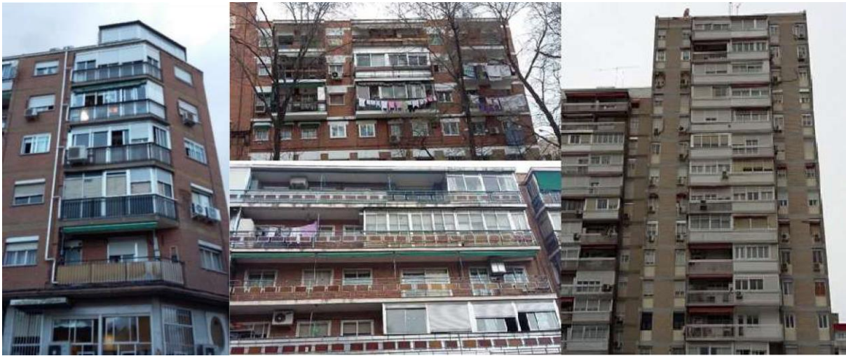
Figure 5.51. Examples of disorderly and irregular balcony enclosures. In the right-hand example, the percentage of enclosed balconies is such that it has become the norm, forming a central body of miscellaneous glazed galleries.
